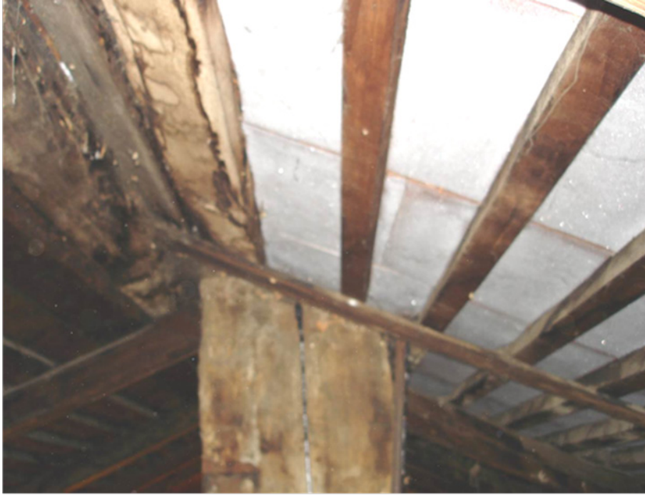
Fig. 8. Condition of the paving elements of the truss system
